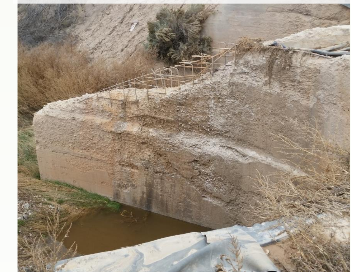
2019 – needing serious repair
