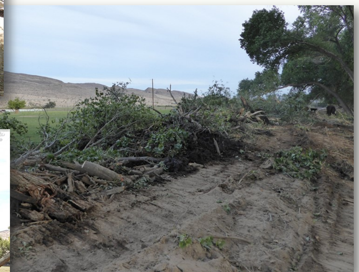
Conservation Camp crews removed live trees and woody material in the drain channel and sawed up the pieces of wood into 4 to 6 feet segments.
