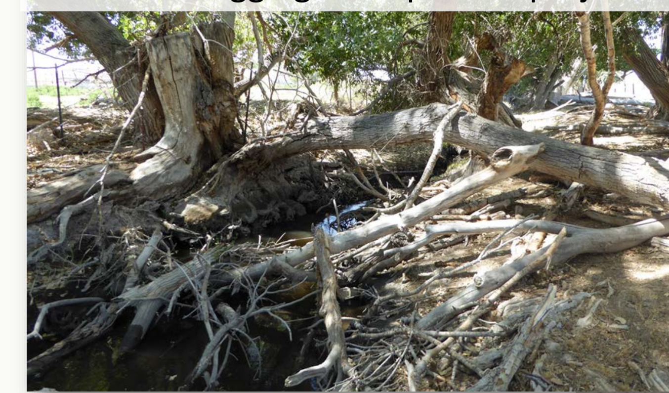
Debris clogging drain prior to project
